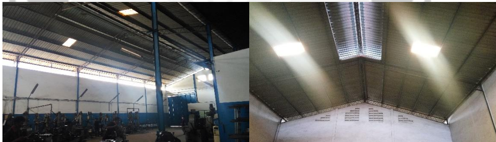
Figure 4.4 Lighting in Production Floor
