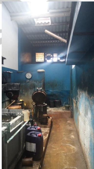
Figure 4.26 Exhaust Fan in Coating Room
