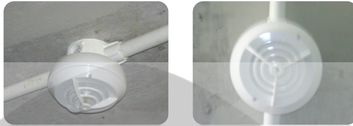
Gambar: 5.21 Fire Alarm
