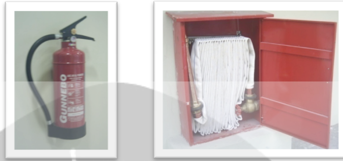
Gambar: 5.19 Portable Fire Extinguisher, dan Hydrant box
